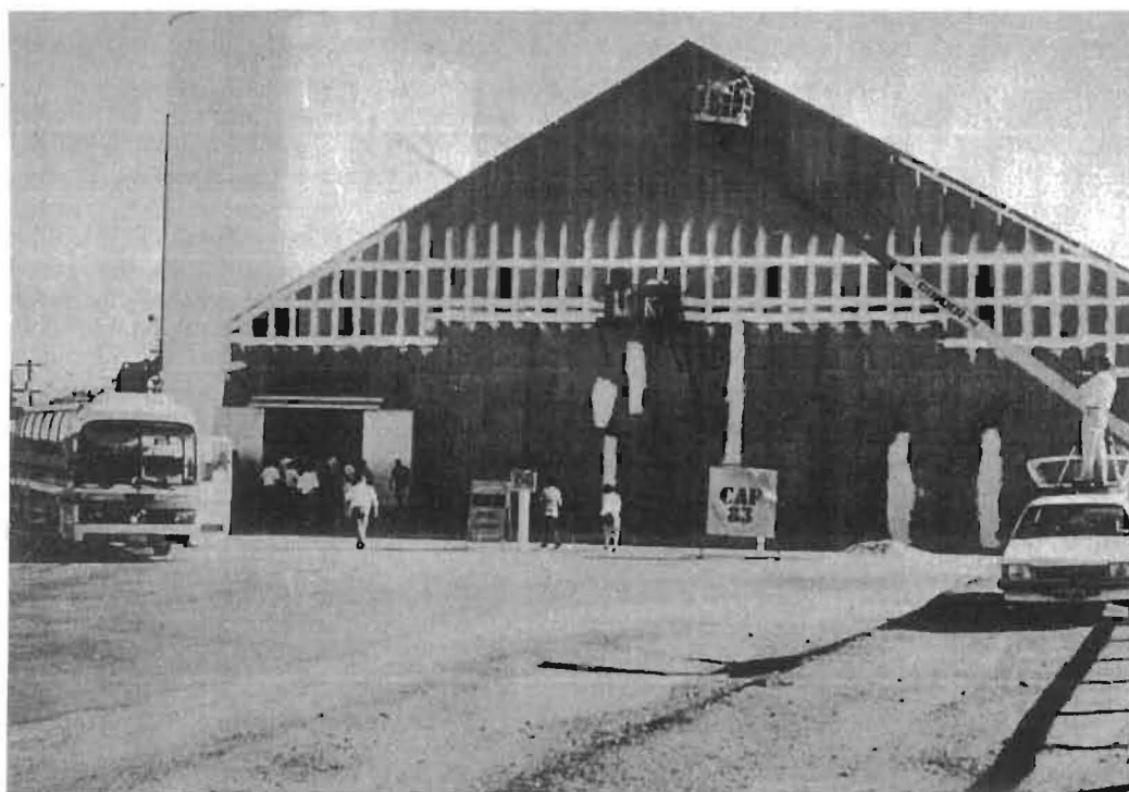
Photo 4. Sealing in progress on the end wall of a horizontal silo at Meckering. Note all lap ends of the corrugated iron sheets used to clad the gable-end wall are individually sealed, as are surface cracks evident in the concrete wall.
