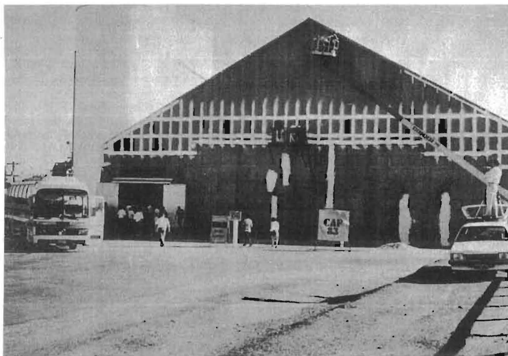
Photo 4. Sealing in progress on the end wall of a horizontal silo at Meckering. Note all lap ends of the corrugated iron sheets used to clad the gable-end wall are individually sealed, as are surface cracks evident in the concrete wall.
