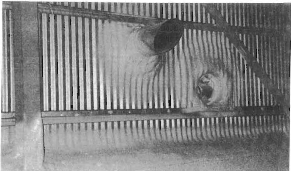
Photo 10. Foam application along an inside wall ledge and around the fan and pressure release duct fitted into a gable and wall.
